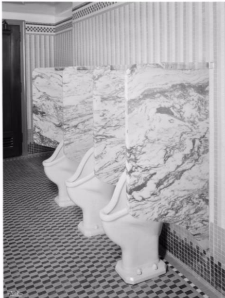
Image 9. The men's toilets at the Texas Oil Co. office in their original condition. 60
